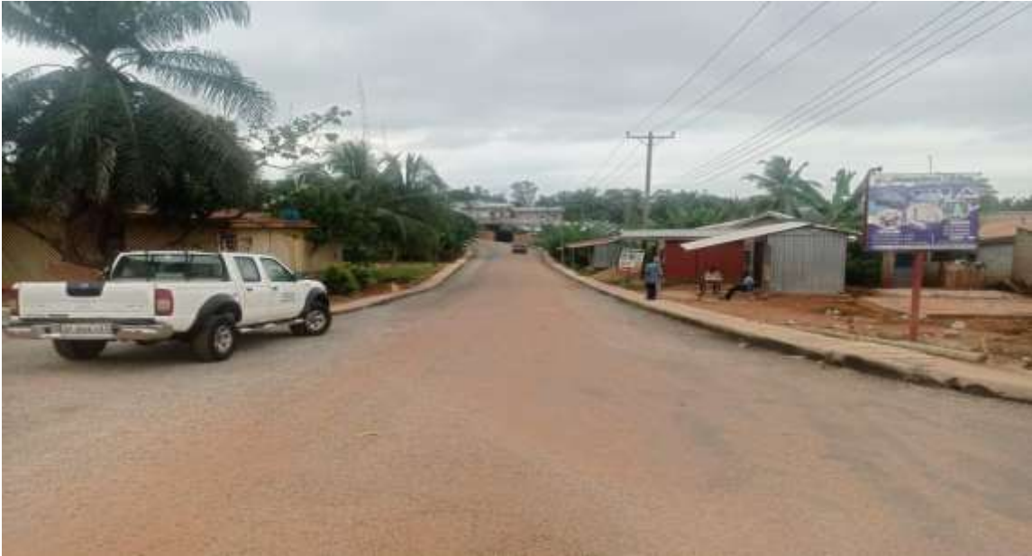
Completed of Bitumen surfacing on Falco Street & Eduful street in Agona Swedru
